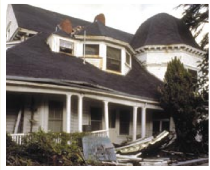
This turn-of-the-century wooden residence sustained major damage when it moved off its foundation during an earthquake.
